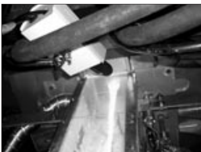
View of glass being drained from the bottom of a cold-crucible melter installed in NETEC for the development of low-level waste vitrification technology.
