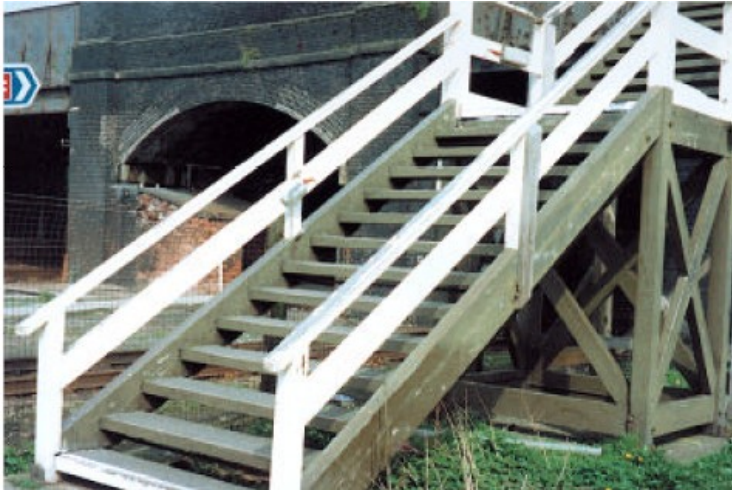
Photo 7. Open tread stairs are a hazard for many disabled people and should not be used
