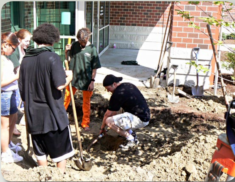
Students preparing the area for The Met's "Dynamic Theatre" statue in front of the Media and Arts Centre at the Public Street campus
