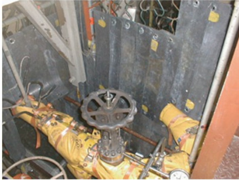
Installation of biological shielding on a pipe enabling monitoring of a valve
