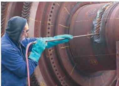
▶ Segmenting large plant items during the dismantling of the cooling towers for residual heat removal. Caorso nuclear power plant, Italy. [Photo: SOGIN]
