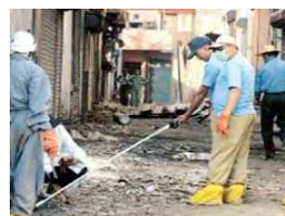
Radiation fields brought down from 0.5mSv/hr-1mSv/hr to 15µSv/hr at the entrance door where majority of sources were found.
