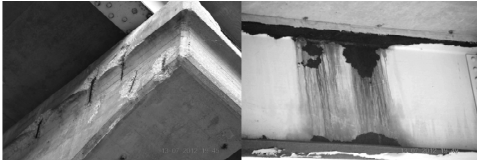
Figure 2.11. Steel and concrete bridge component corrosion
