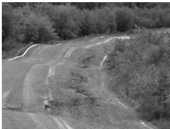
Figure 2.7. Melting permafrost: Heave damage to roadway
