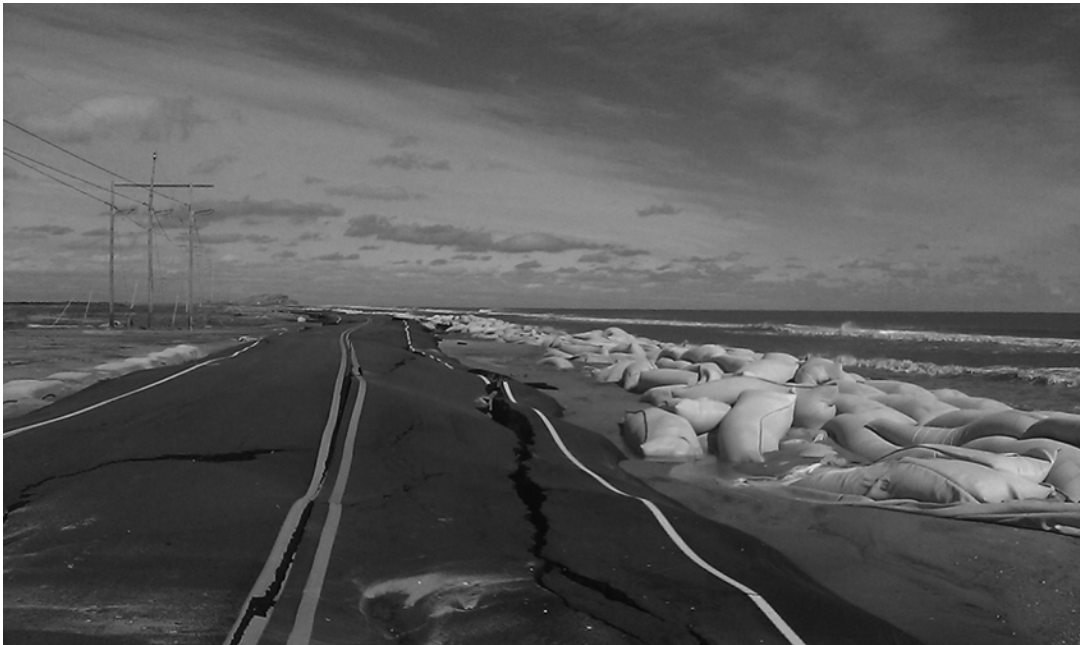
Figure 2.8. Hurricane Sandy storm-surge damage on Highway 12 in North Carolina
