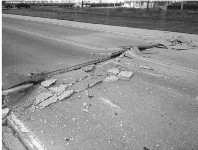
Figure 2.6. Concrete slab pavement blow-up due to elevated heat and base humidity
