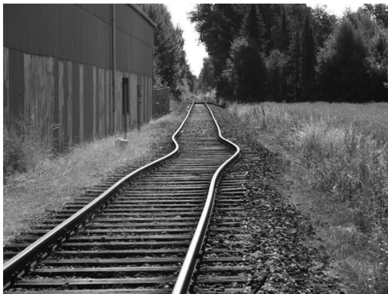
Figure 2.18. Heat-induced track buckling
