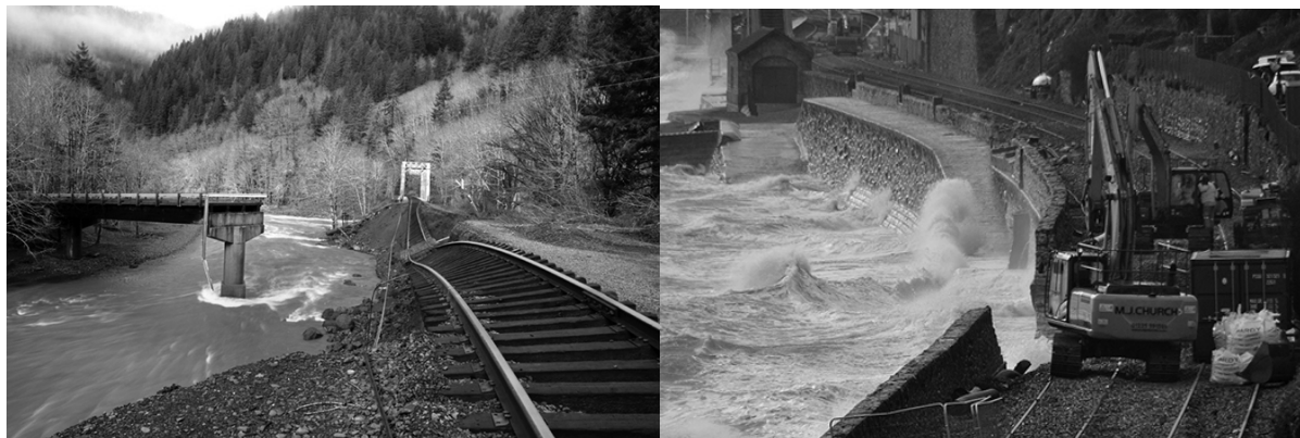
Figure 2.16. Impacts of storm-related embankment scour
