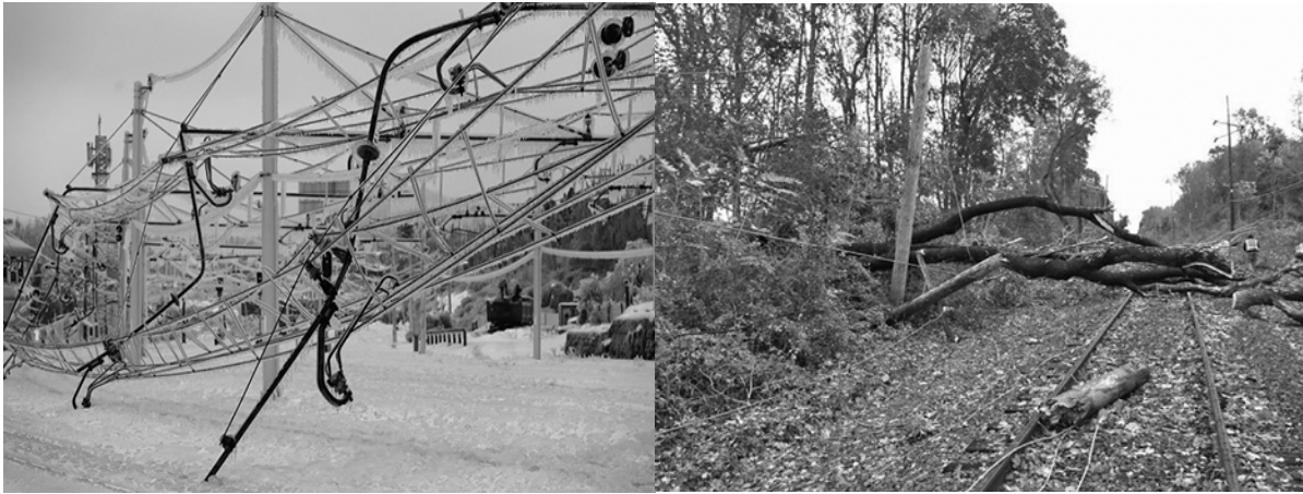
Figure 2.19. Ice damage to rail overhead structures and storm-fall on rail tracks
