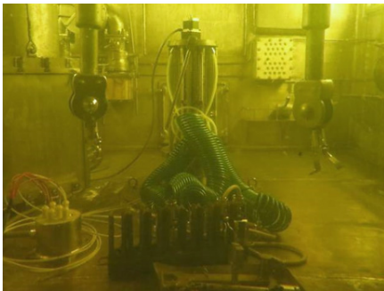
Figure 2.121. Zn Decladding unit in hot cell during experiment
