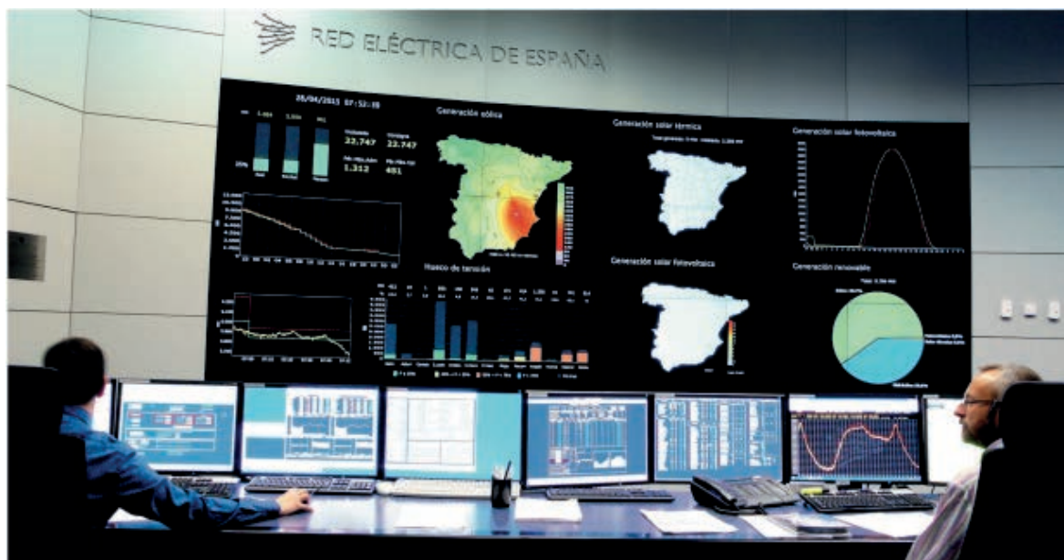
Figure 3.8 • CECRE's control room
