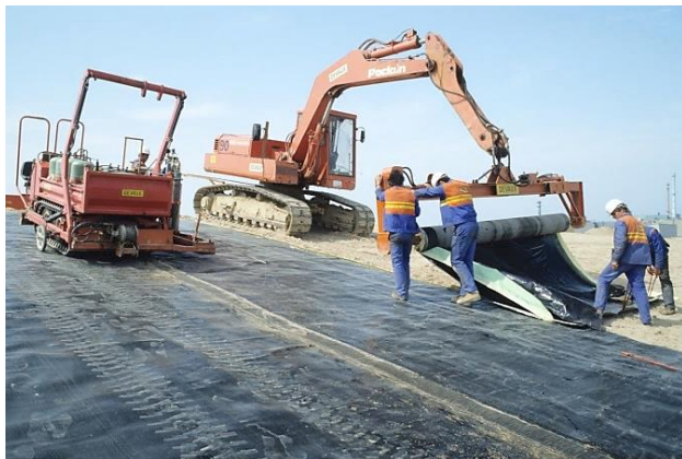
Laying a geomembrane strip. The strips are welded to each other along an axis parallel to the north-south axis.
