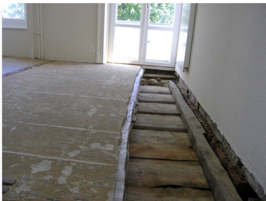
Figure A3.17. Photo of the remediation of a contaminated room with partial removal of floor coverings
