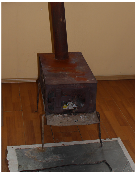
Boiler in a kindergarten in the Marneuli region, © Energy Efficiency Center, Georgia
