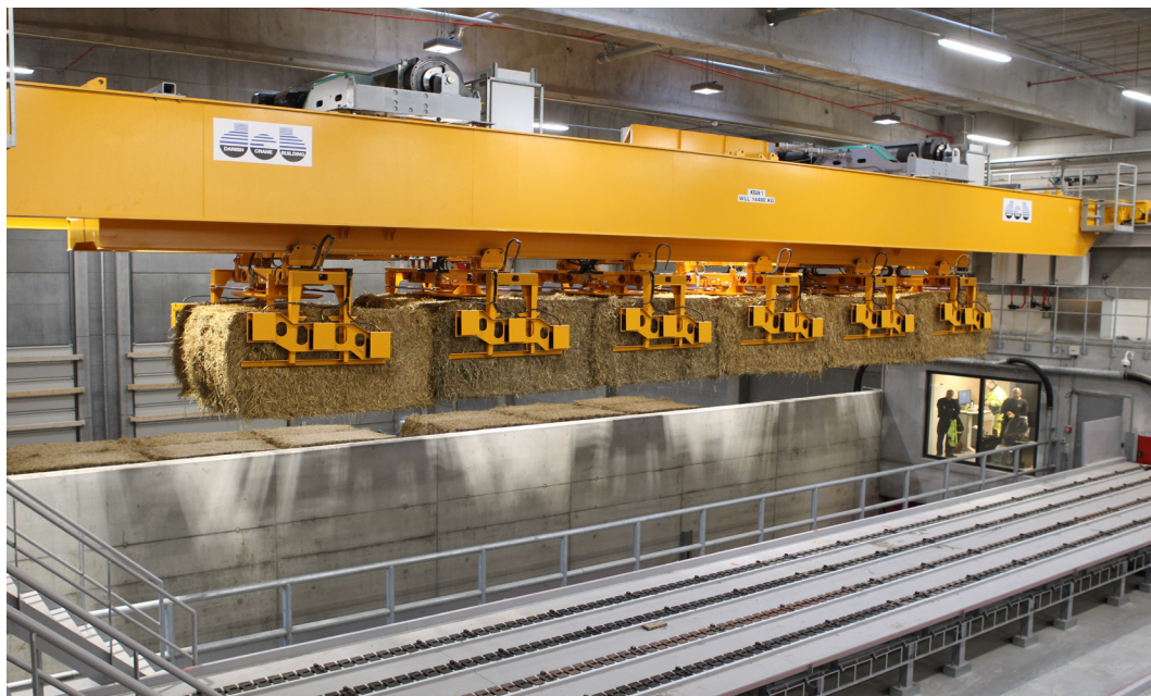
Straw boiler plant (© AffaldVarme Aarhus)
