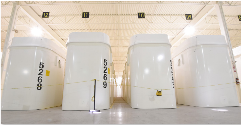
Figure 3.6. Spent fuel dry storage containers in Canada
