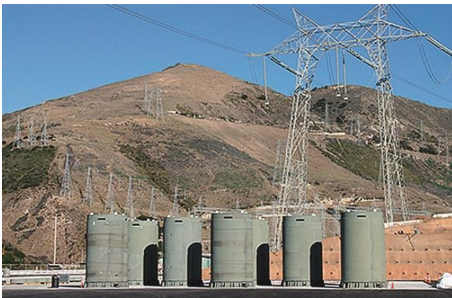
Figure 3.7. Dry storage facility for spent fuel in the United States
