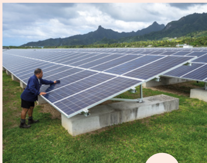
The solar panels are regularly cleaned at the Rarotonga International Airport, the Cook Islands.
